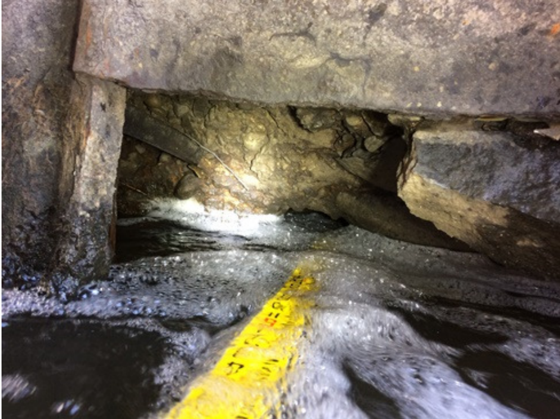
Photo 4 – Looking below the bottom of the sheet piling and into the void beneath the footing of Abutment 1.
