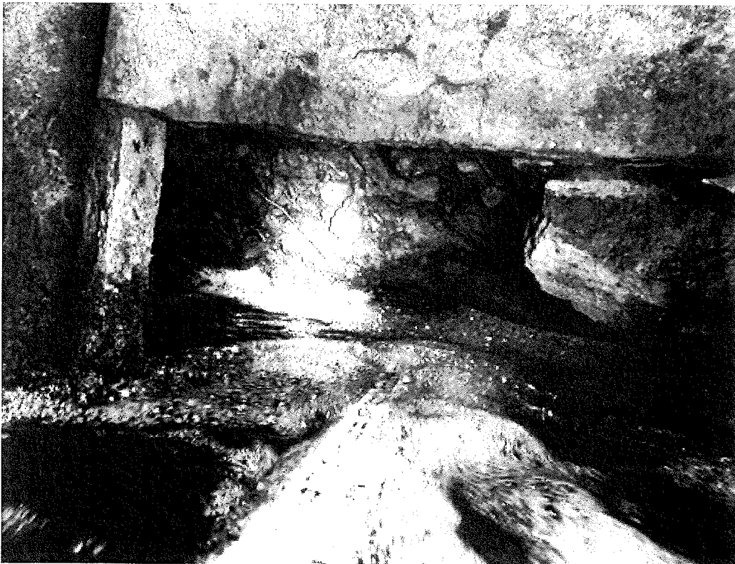
Photo 4 – Looking below the bottom of the sheet piling and into the void beneath the footing of Abutment 1.
