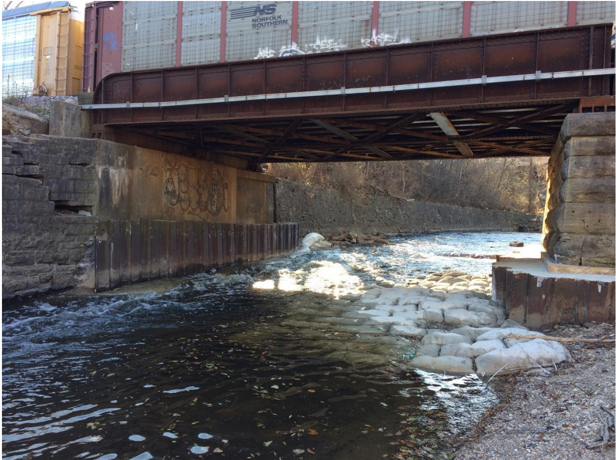
Exhibit 2: The photo is looking southeast at Abutment 1 and Span 1 of Watertown BR 88.74 and shows the project site after placement of the grout bag mat.
