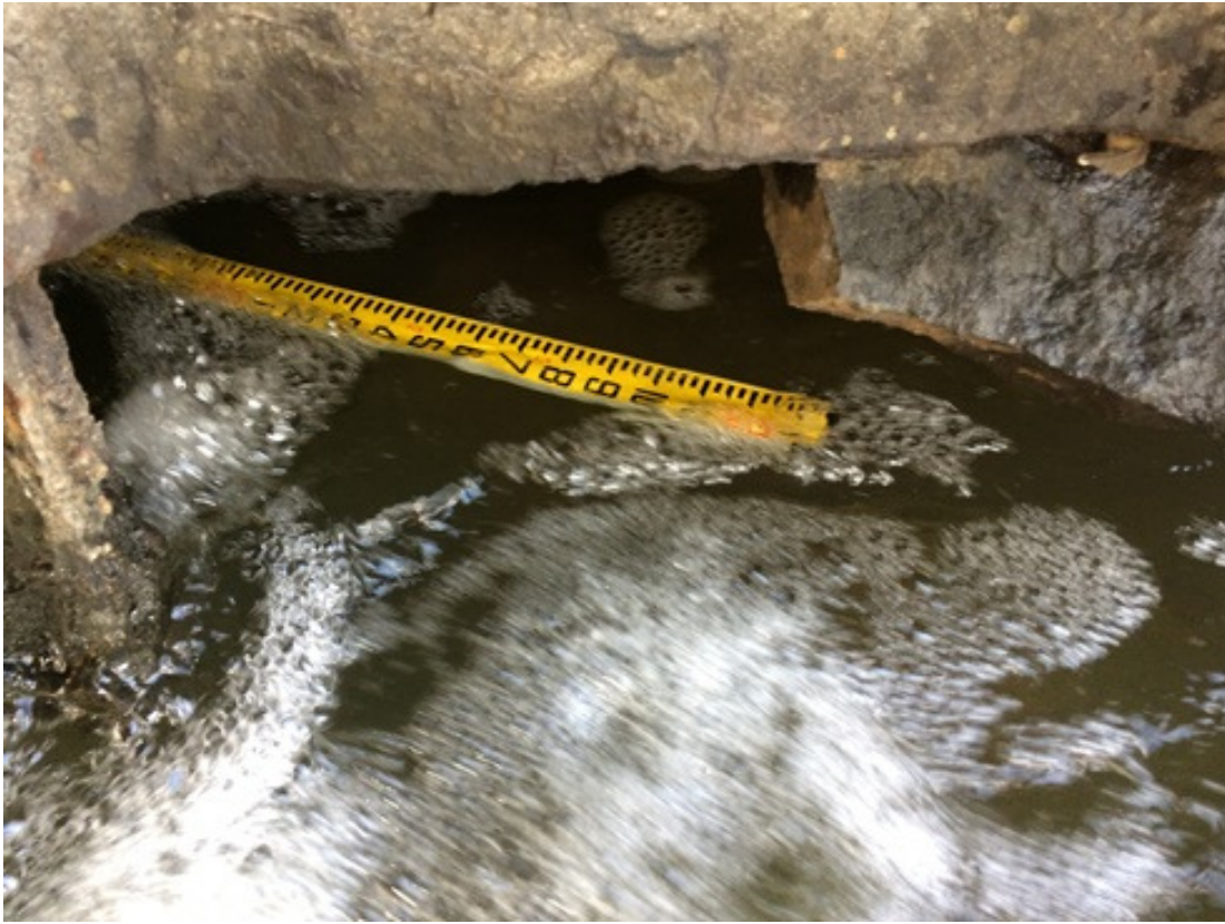
Photo 5 – Full extension of 13’ long tape measure under the Abutment 1 footing.
