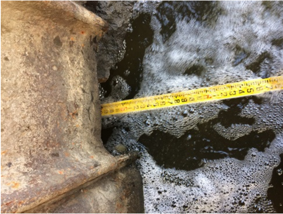
Photo 3 – Tape measure extended 5' beneath footing of Abutment 1.
